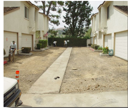
Right: 100 block of Mountain Ct. viewed from Park Lane. Country Road men work on underground electrical conduit disrupted during asphalt demolition.
